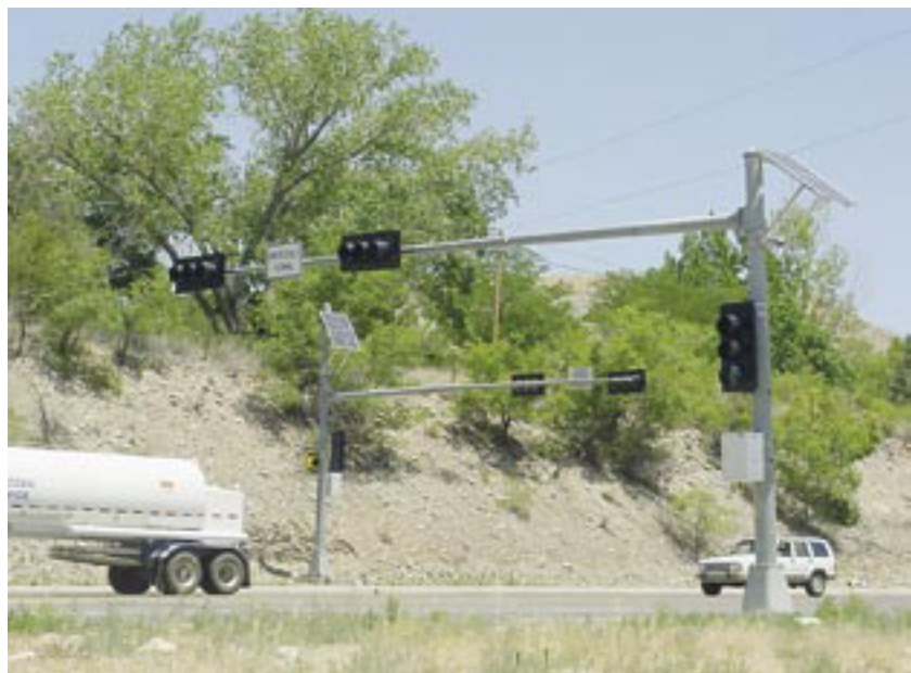
Three 3-section signal heads (solar powered). Lights are green until fire station activates.
